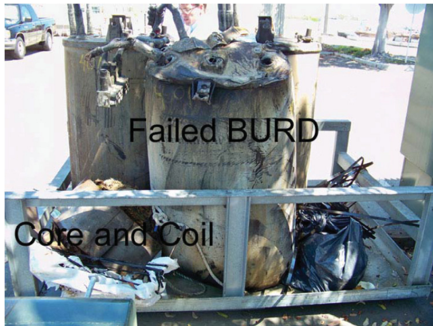
Figure II-5 – D1b (BURD Transformer): Catastrophic Failure
